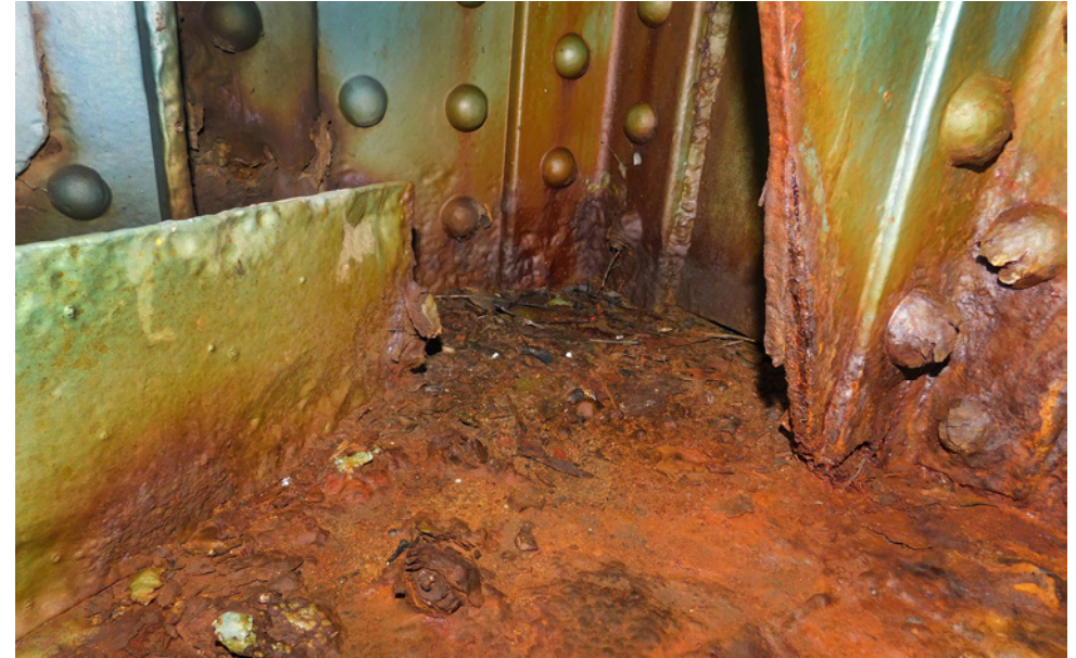
Obr. 3.122. Detail stavu NK nad pilířem P2 (HPM, Pontex) Fig. 3.122 Detail of the condition of the superstructure above the pillar P2 (HPM, Pontex)
