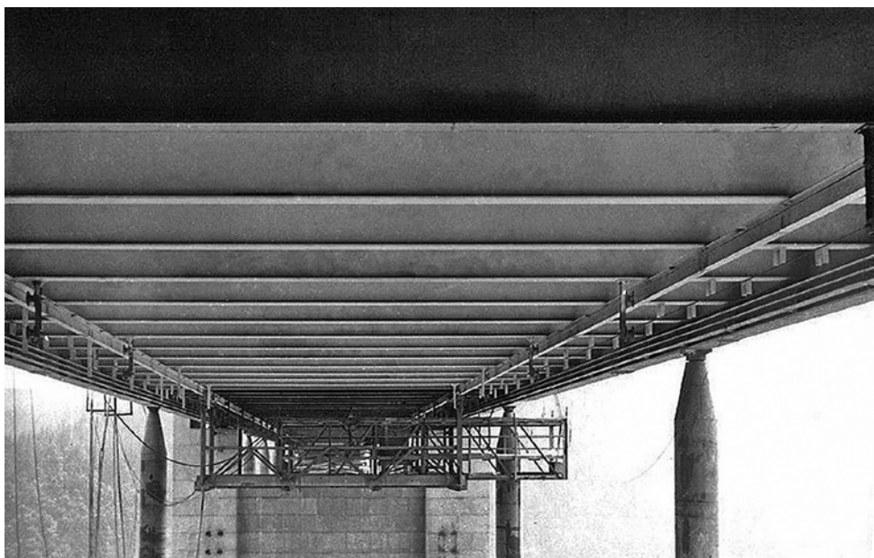
Obr. 1.41. Žďákovský most – pohled zdola na mostovku (1967) Fig. 1.41 Žďákov Bridge – view of the bridge deck (1967)
