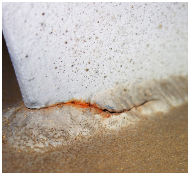
Obr. 3.140. Trhлина ve svaru Fig. 3.140 Crack in the weld
