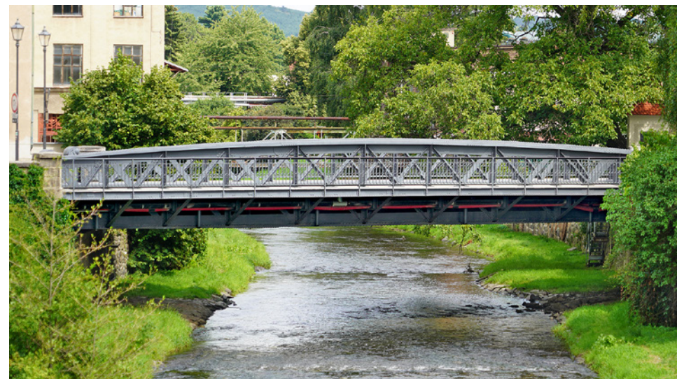
Obr. 3.94. Pohled na most od jihozápadu Fig. 3.94 View of the bridge from the southwest
