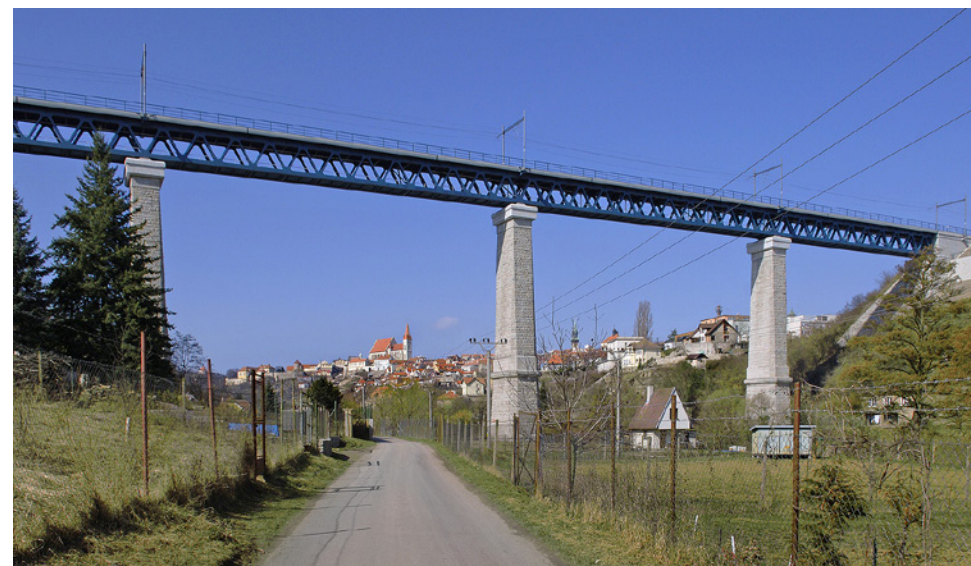
Fig. 1.27 (a, b) Truss deck-type bridge with straight chords (railway bridge in Znojmo from 1871 and after reconstruction in 2009)
