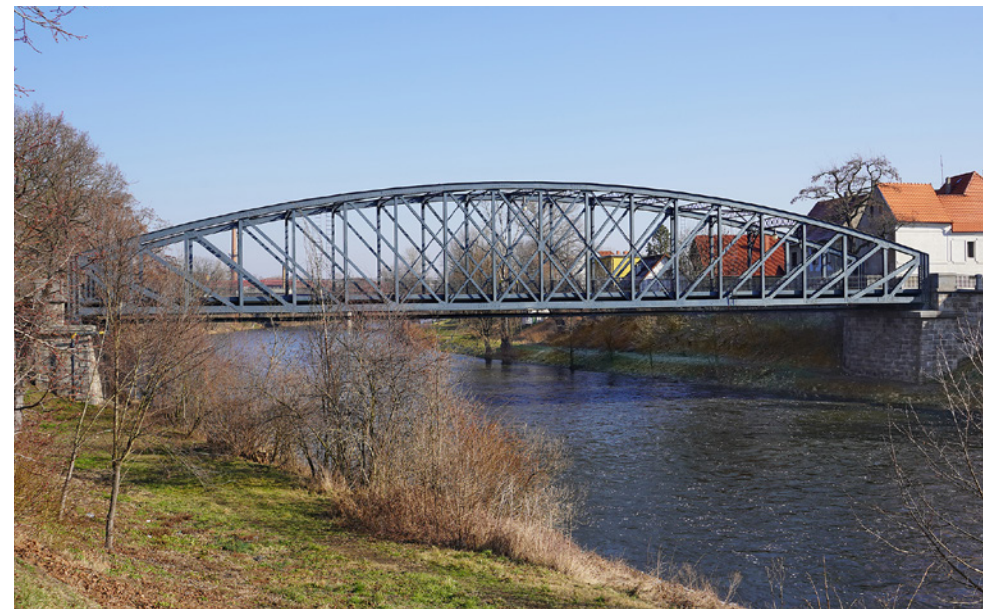
Obr. 3.85. Pohled na most od jihozápadu v roce 2020 Fig. 3.85 View of the bridge from the southwest in 2020
