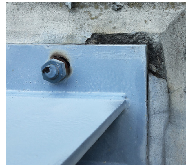
Obr. 3.142. Porucha šroubu u kyvné stojky Fig. 3.142 Bolt defect at the double-pinned strut
