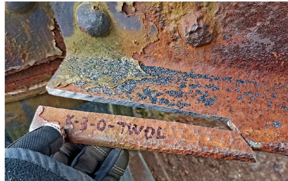
Fig. 1.50 Example of intervention into historic structure according to invasiveness of survey. b (a) Non-invasive survey – hardness test (a) Invasive survey – specimen for tensile test
