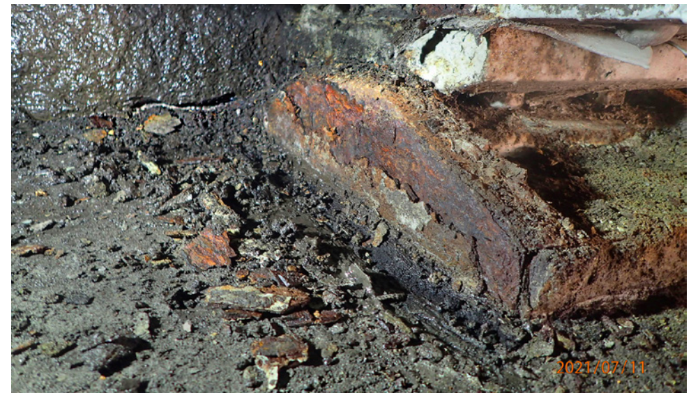
Obr. 3.37. Degradace a koroze ložisek Fig. 3.37 Degradation and corrosion of the bearings
