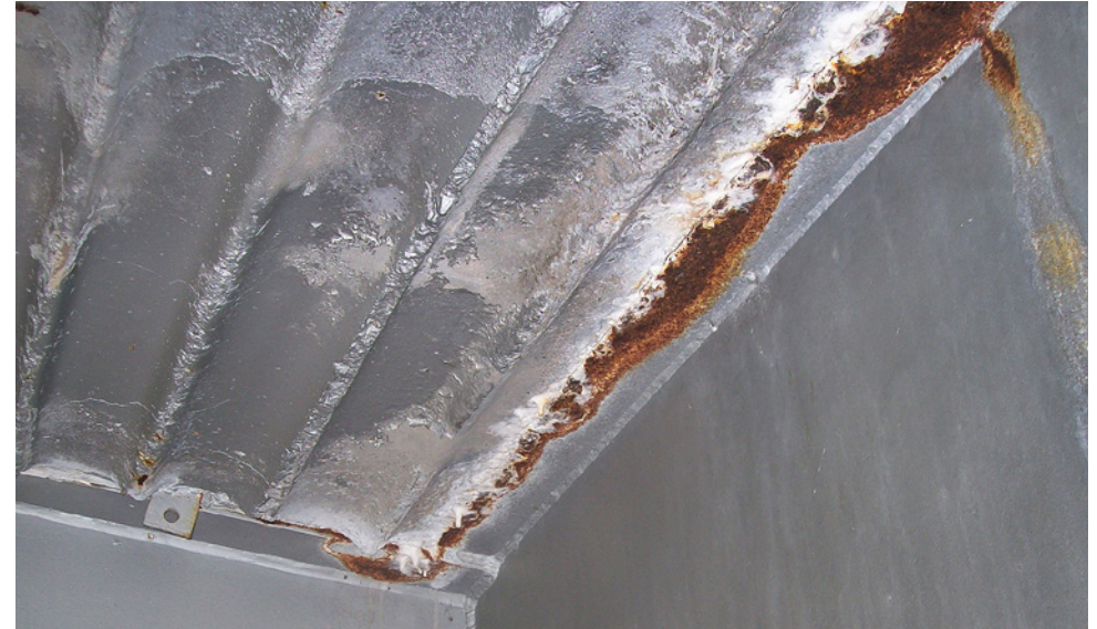
Obr. 3.162. Pohled na desku mostovky zdola Fig. 3.162 View of the bridge deck from below
