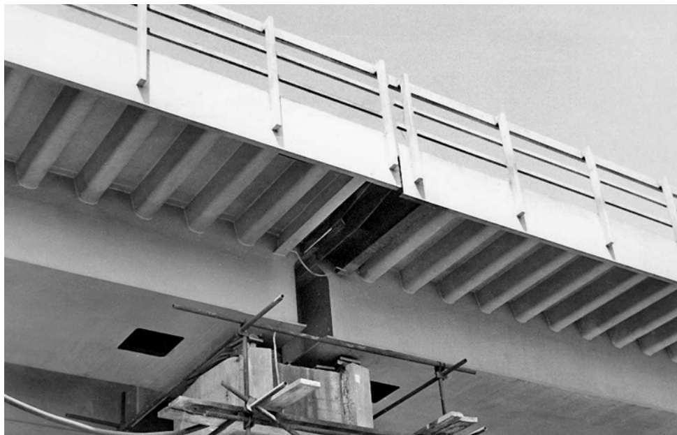
Obr. 1.43. Severojižní magistrála – spojení mostovek s tepelnou dilatací (1978) Fig. 1.43 North-South Main Line – connection of bridge decks with thermal expansion of the roadway (1978)
