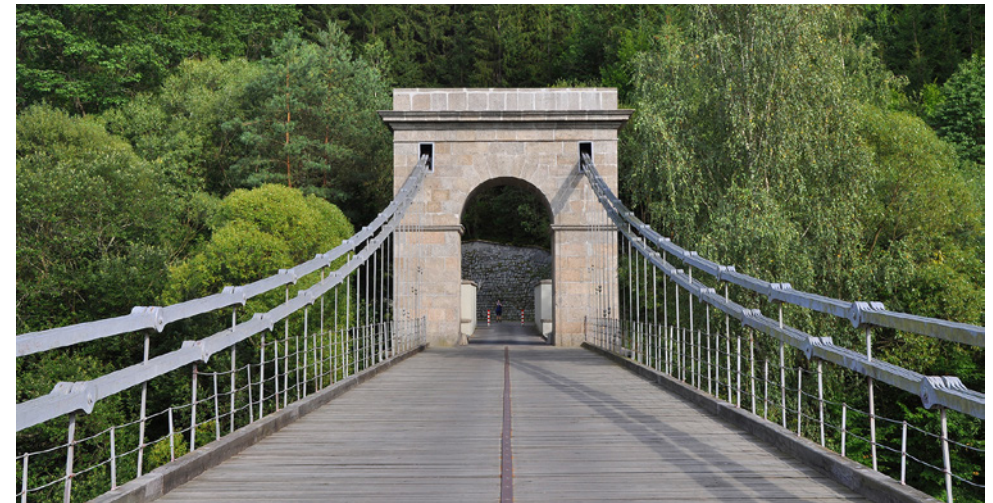
Fig. 3.58 View of the bridge deck, chains and pylon in 2019 (photo: authors' archives)
